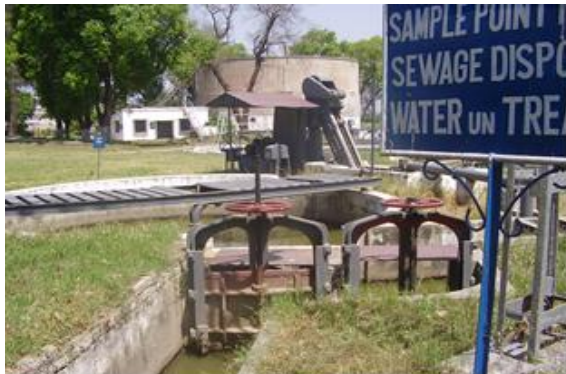
Figure 2: Entrance point of Raw Sewage in Treatment Plant
