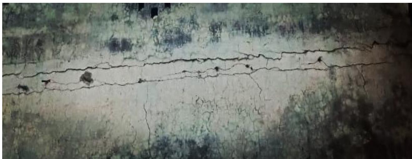
Figure 1: Building affected due to ASR
